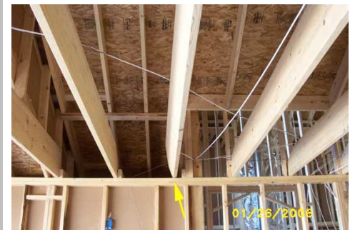
Looking east @ garage interior east side – note arrow points to severe twisting ceiling joist 9
