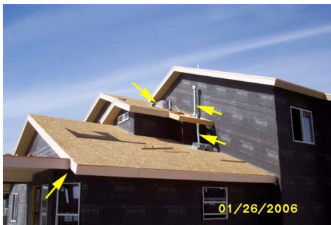
Looking @ south east corner of house – furnace and water heater flues too short and too close to vents and AC 7
