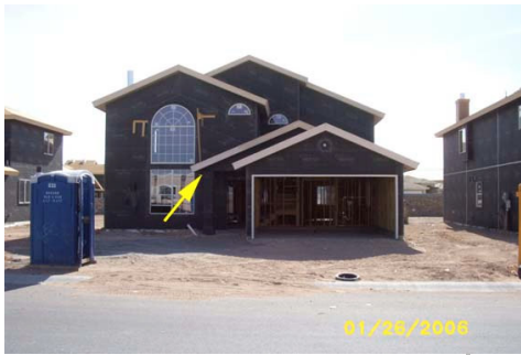
Looking south @ front of house – note arrow indicates missing stucco lathe (mesh) 1
