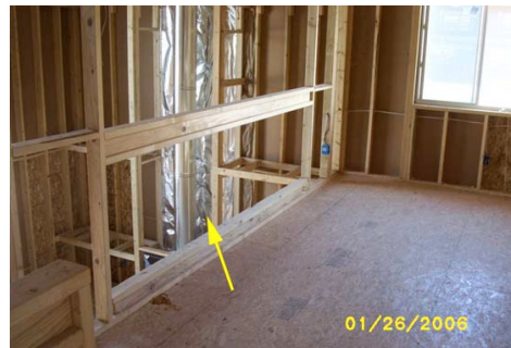
Looking @ railing in loft over looking living room – note no presence of vertical balusters 11
