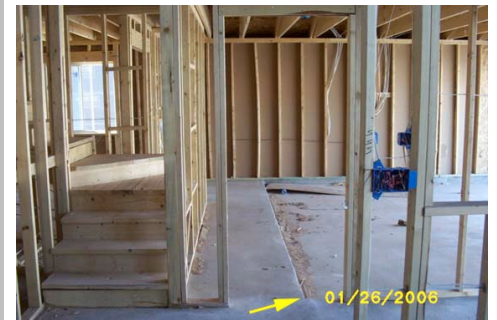
Looking @ door leading to garage – note garage step down bisects pathway in and out of door 12
