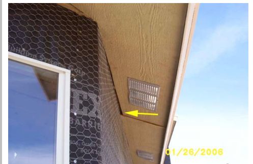
Looking north @ gap along east side soffit 6
