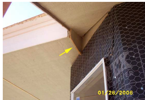
Looking southwest @ east side porch transition to house – note problematic transition 5
