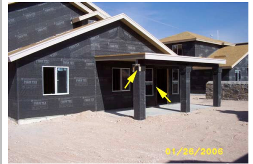
Looking north east @ rear of house – arrows indicate missing column caps and indicates missing stucco lathe 3
